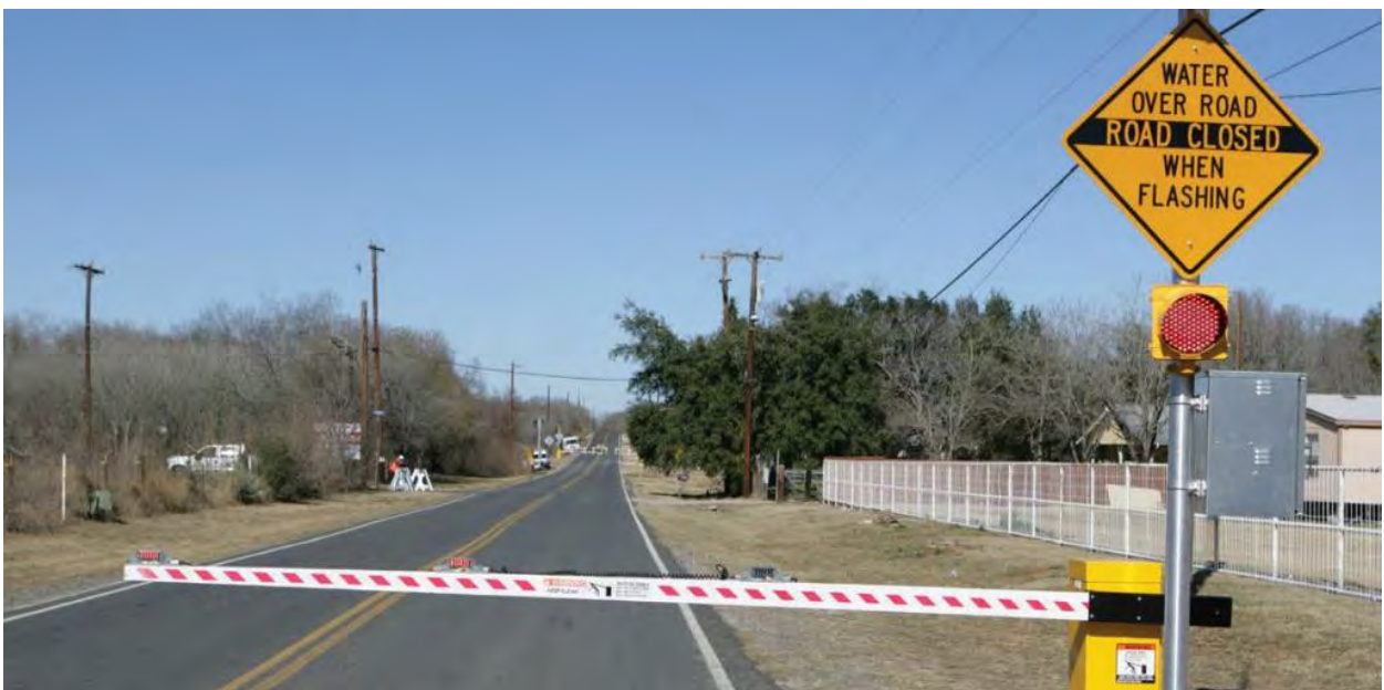
Figure 65 - Flood Detection System Automated Gate Example
