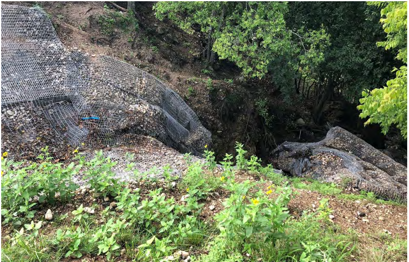
Figure 37 – Channel Failure at Guadalupe River Bank
