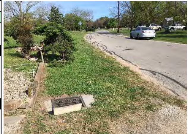
Existing Undersized Drainage Network at Jack Drive
