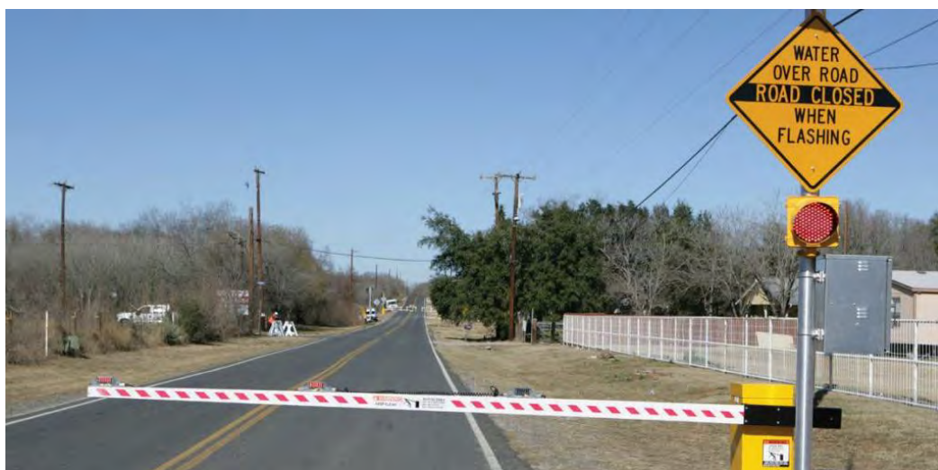
Figure 63. Flood Detection System Automated Gate Example
