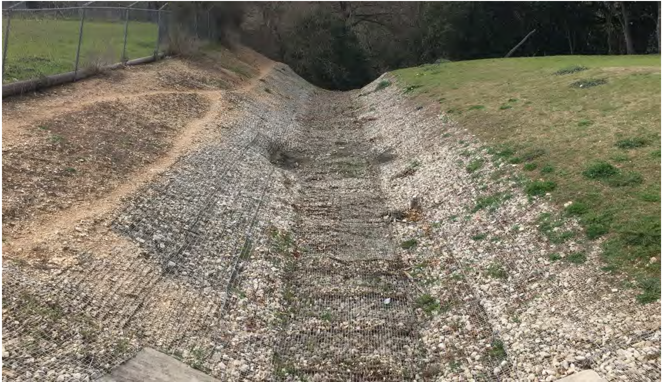
Figure 36 – Channel Erosion at Spring Street
